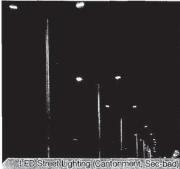
LED Street Lighting (Cantonment, Secbad)
